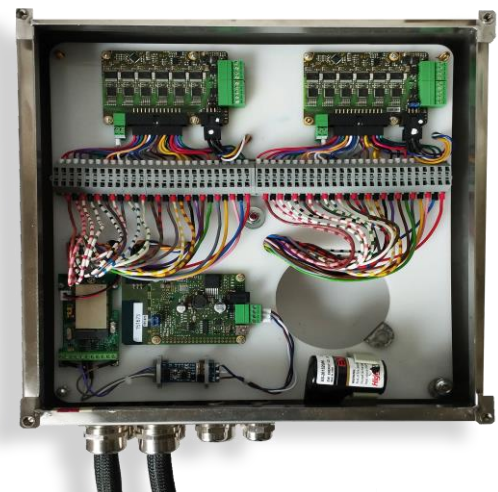
Fig.1 Cell voltage monitoring unit
